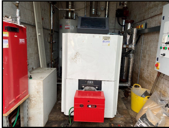
Single oil boiler
